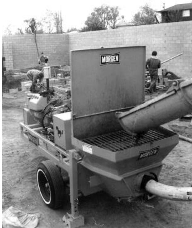
Fig. 4—Pump with hydraulically powered valve
