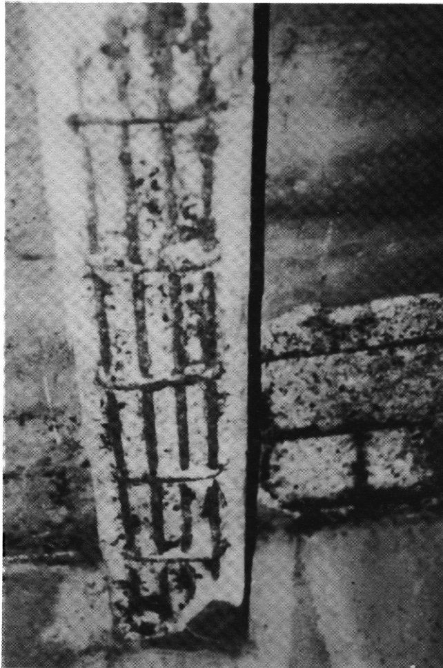
Fig. 1.8-Spalling of beam soffit beside leaking isolation joint
