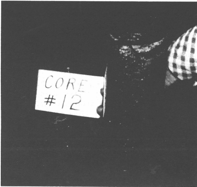
Fig. 1.4-Core showing top delaminations
