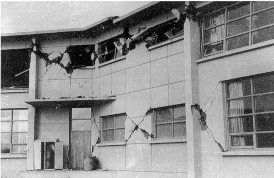
Figure 6-15. Damage concentrated at the intersection of two wings of an L-shaped school, Anchorage, Alaska, 1964
