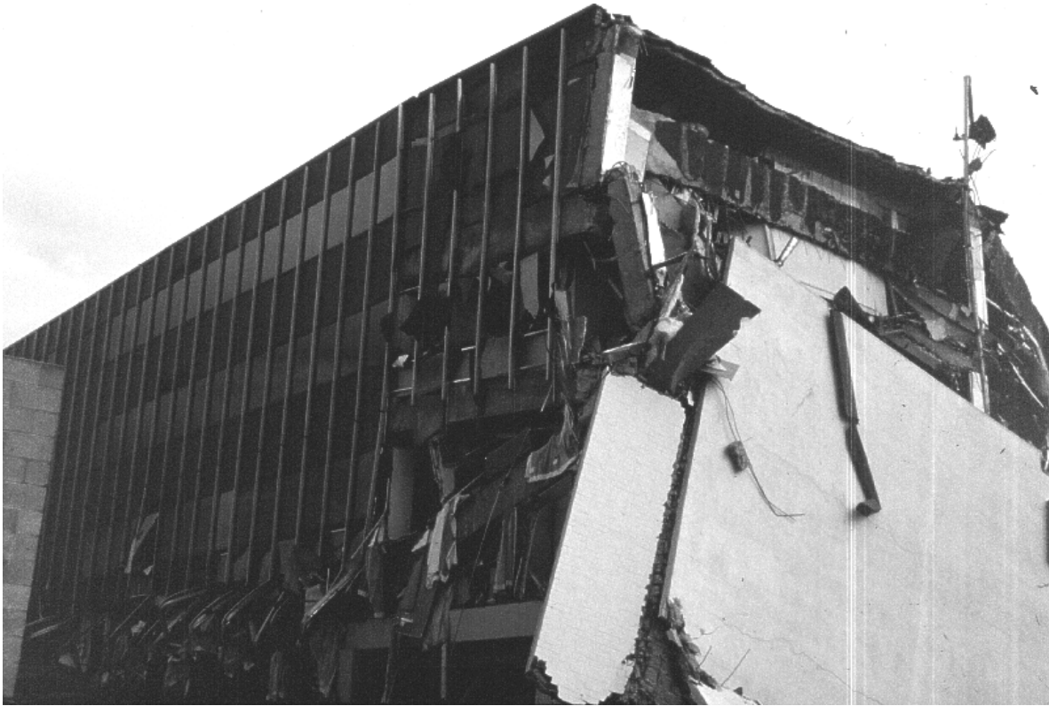
Figure 6-31. Discontinuous shear wall failure, office building, Northridge
