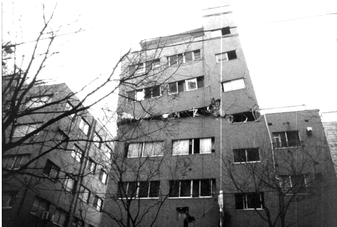
Figure 6-38. Failure of set-back building along a plane of weakness
