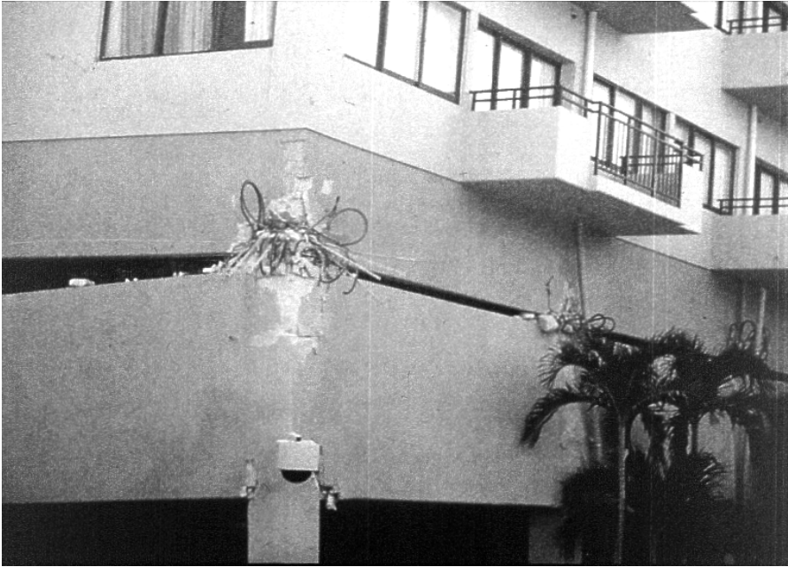
Figure 6-34. Short column failure, Guam, 1993
