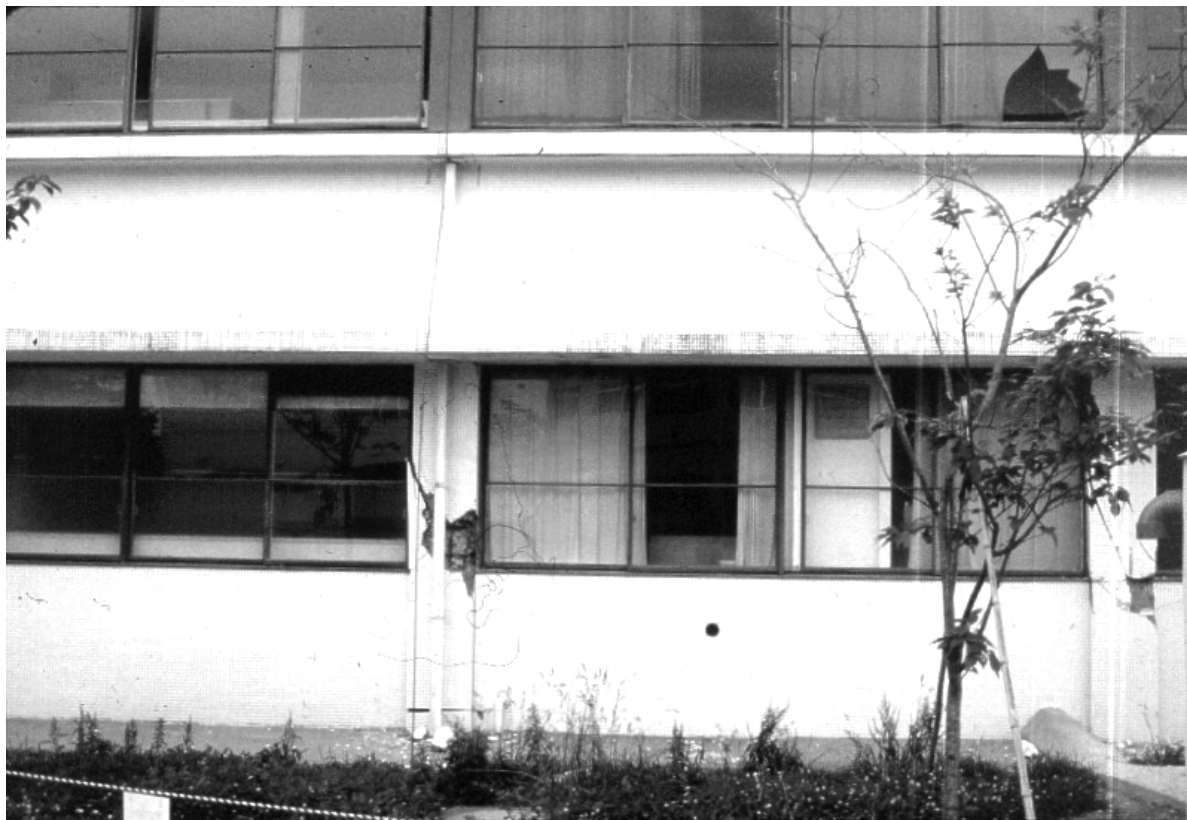
Figure 6-33. Short column failure, school, Japan: Miyagi-ken -oki, 1978
